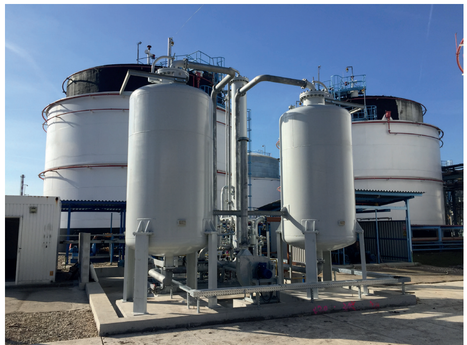
Figure 6 – Vapour recovery unit based on activated carbon and absorption. Cool Sorption, 2019
